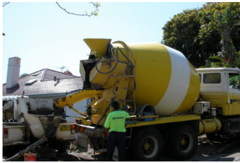
The concrete for the ground floor slab has arrived and is being pumped.
