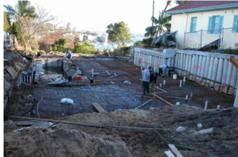
Steel reinforcement and plumbing in place for the placement of the lower ground floor concrete.
