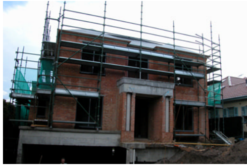
The scaffolding is in position, ready for the external finishes to be applied.
