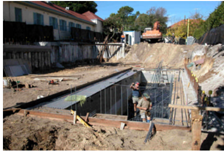
Construction of the “indoor” pool has begun with formwork done and steel fixing. Note the concrete and reinforcement to the right of the pool. The concrete is part of a contiguous pile wall required to retain the neighbouring property during the construction of the pool.
