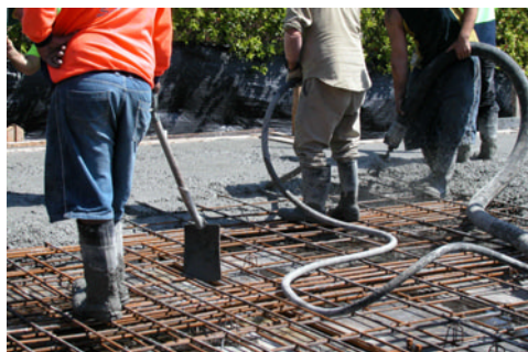
Concrete pump/placement on right. Vibration/compaction in the middle. Man leaning on shovel on the left. When working the shovel bearing person assists in levelling the concrete for the screeder (or finer levelling) level the concrete.
