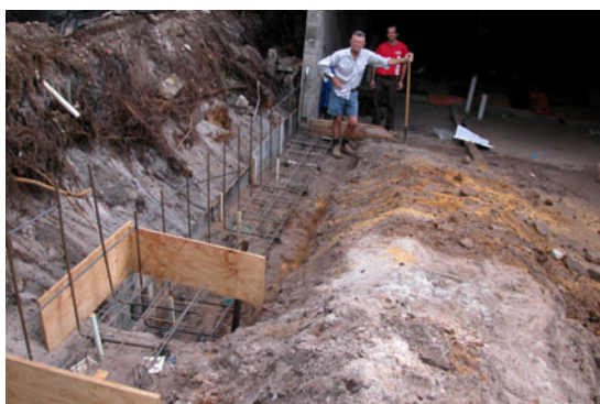
Footings and reinforcement for the concrete block retaining wall ready to go.
