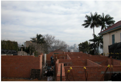
Lower ground floor walls complete and ready to accept the ground floor slab.
