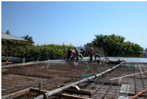
Concrete placement for the ground floor is well under way. Note the steel tube that carries the concrete into position.
