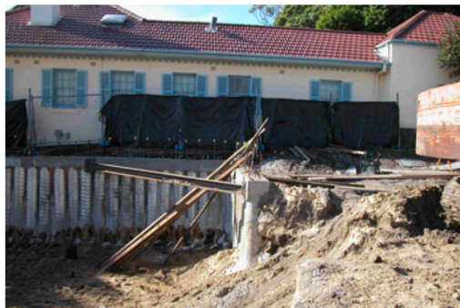
Steel strut is installed to brace wall. The brace provided efficiently through a shallower pile depth.
