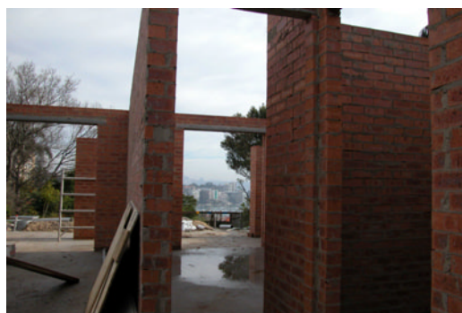
The lower ground floor slab is poured, brick work is under way.
