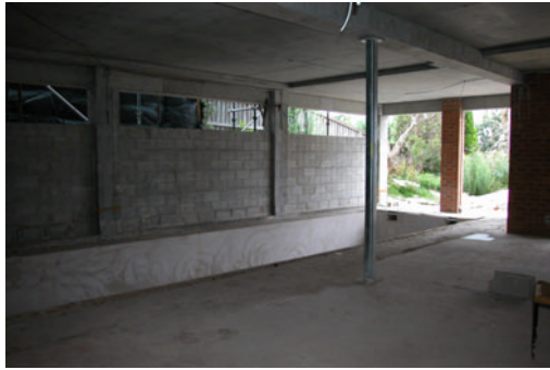
Lower ground slab complete, ground floor complete cover and the indoor pool evident in the brick ground.
