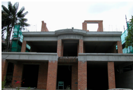
Rear elevation – all floors now in place. The brickwork for the first floor is underway.
