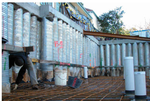
Steel fixing. The location of the steel reinforcement within this depth of the concrete is paramount.
